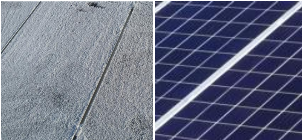
Figure 12. View of the module surface covered with snow after partial (left) and complete snow removal (right).
