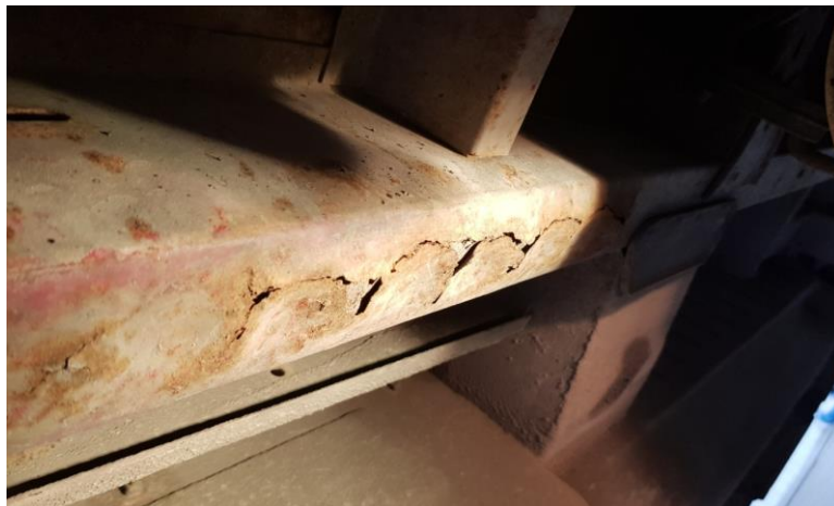
Figure 3. A photograph showing a vehicle chassis structural element in an advanced state of degree of erosive corrosion.
